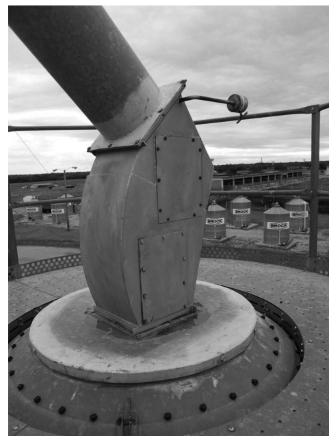
Figure 13. Fill spout equipped with a self-closing door to reduce leakage up the leg. Seam where fill spout attaches to top of the bin needs to be caulked also.
