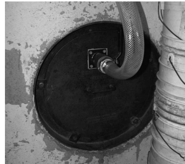
Figure 3. Manhole cover in concrete silo with CLF injection point and ball valve to isolate bin.
