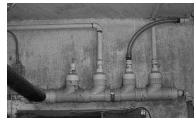
Figure 7. PVC distribution manifold for CLF system.
