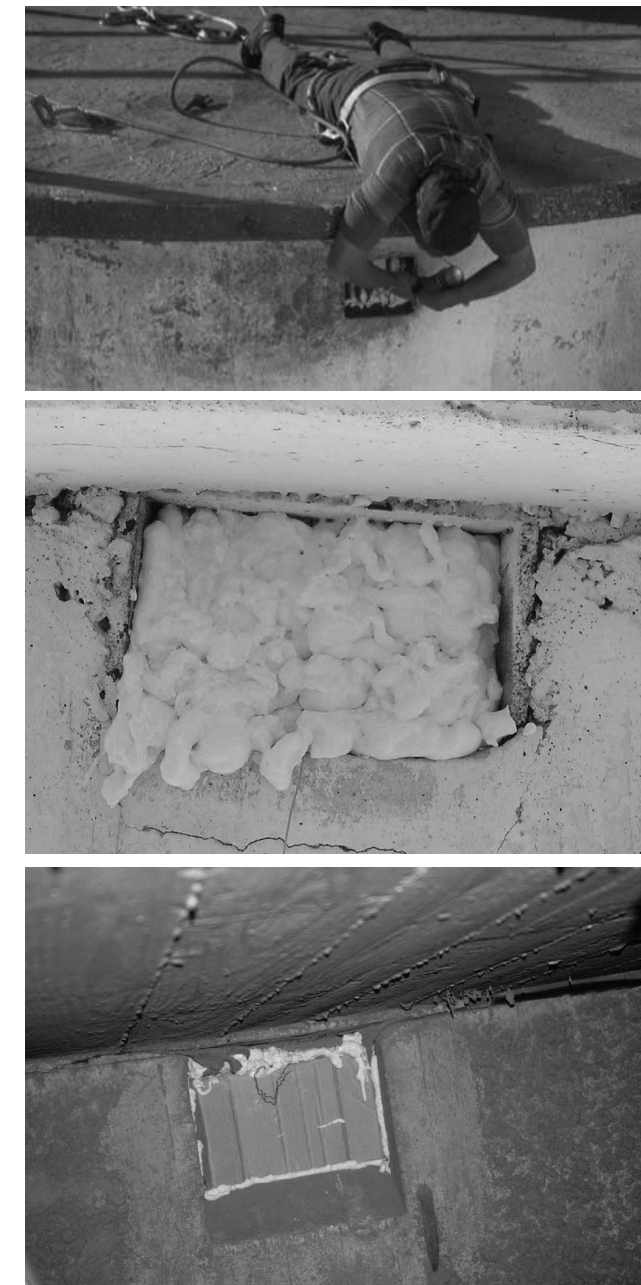
Figure 8. Sealing concrete silo top vents with closed cell expandable foam. Interior cardboard support is temporarily held in place with wire while foam is applied from outside.
