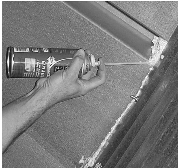
Figure 9. Bin roof and sidewall seam sealed with silicone caulk and closed cell foam.
