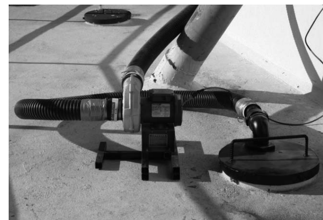
Figure 5. CLF fan pulling gas through manhole cover on top of concrete silo. Flexible corrugated drain hose is used for temporary connections.
