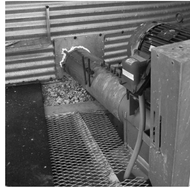
Figure 14. Unloading auger with permanent sealing on bin penetration and temporary sealing on slide gate push rod opening.
