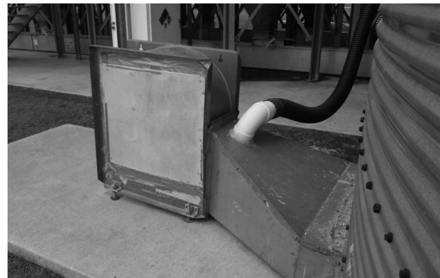
Figure 18. Aeration fan intake sealed with polyethylene film and duct tape. A plywood support panel is secured over the fan opening to protect the polyethylene film from wind damage.
