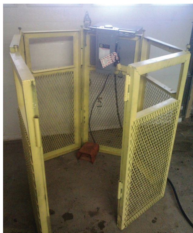
Figure 12. Worker protection caging and sweep auger controls.
