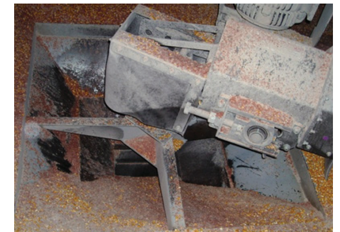
Figure 2. Unguarded bin sump.
