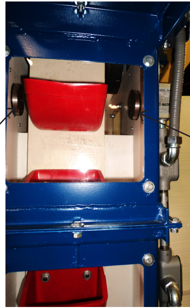
Figure 7: Belt alignment sensors. (Notice the difference in space between the bucket and the sensors on the right and left. The belt is out of alignment.)
