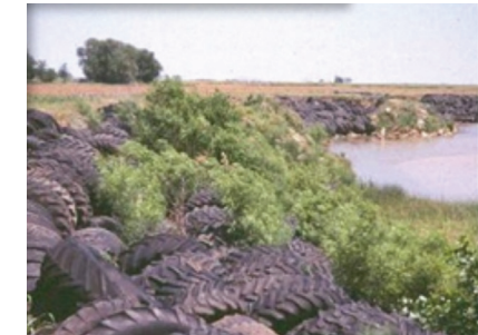
Figure 5. Concrete channel lined with riprap held in place with gabions in Stillwater, OK (A). Tire riprap along the Red River and concrete chunk riprap (B and C).
