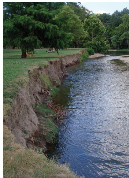
Figure 2. An example of bank erosion and land loss on the Illinois River.
