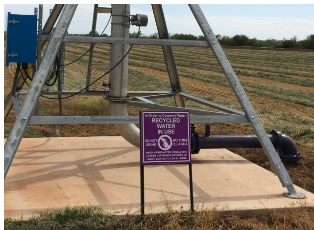
Figure 3. Reclaimed water is used for forage irrigation at the OSU South Central Research Station near Chickasha, OK.
