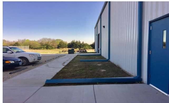
Figure 5. Picture of downspout reconnected to sidewalk (discouraged).
