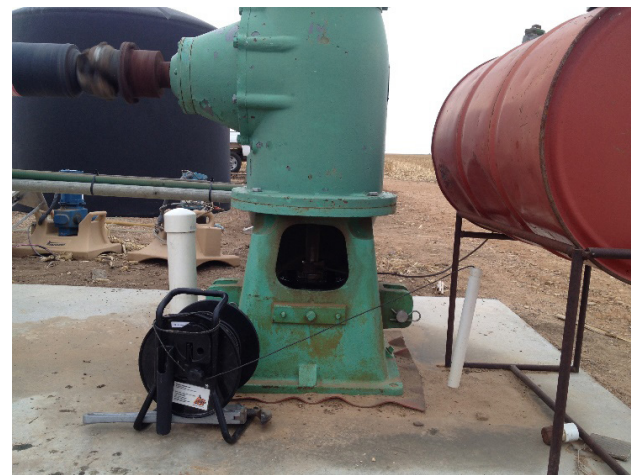
Figure 3. Cable going into well access tube.
