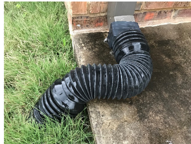
Figure 3. Connecting downspouts with drains can help in routing water away from the foundation of the house to a location better suited to handle the large volume of water deposited on-site during heavy rainfall.
