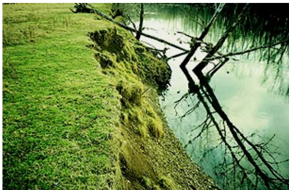
Figure 2. Bank sloughing is a dangerous form of instability that requires attention to the base or toe of the slope. Planting trees at the top of the bank would only worsen the condition.
