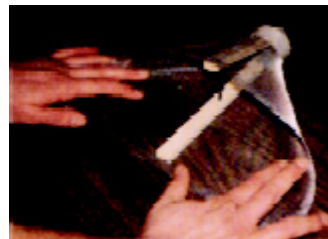
Figure 6G. Anchor dry wall screw into larger piece of wood lath. Do not go through the wood.
