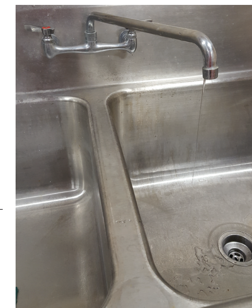
Faucet leak on three-compartment sink in a food-processing facility.
