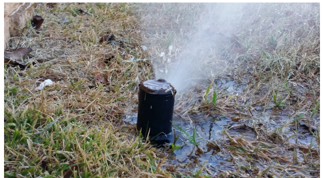
Figure 4. Sprinkler head leaking and causing ponding at the base.
