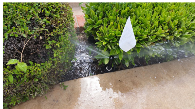
Figure 8. Plants blocking a sprinkler head causing an uneven spray pattern.
