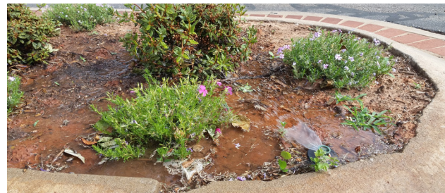
Figure 6. Sprinkler head stuck and failing to fully pop up above the ground.
