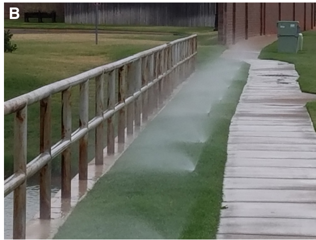
Figures 2a and 2b. High pressure in an irrigation system leads to misting and a reduction in irrigation efficiency. Photos courtesy of Oklahoma City Utilities Department.
