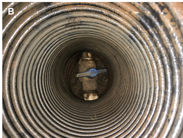
Figures 6a and 6b: The isolation valve is typically located in a small green valve box near the water meter or backflow preventer. This valve is in the closed position. Photos courtesy of Kevin Moore.
