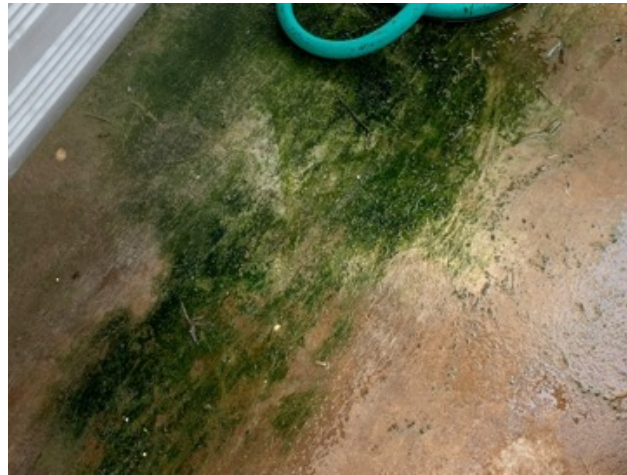
Figure 3. Algae growing beneath a mist bench that can lead to a slipping hazard as well as a site that harbors fungus gnats.
