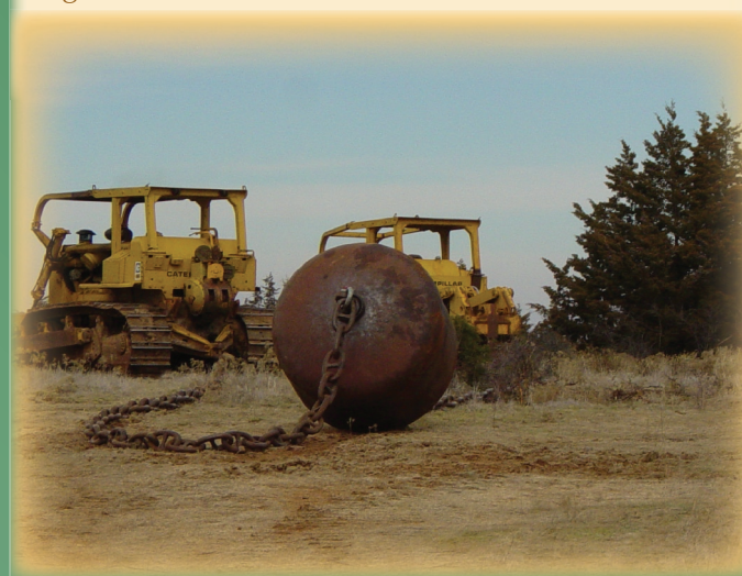
Elevated anchor chains (ball and chain) are the most effective and economical method for eradicating large eastern redcedar.
