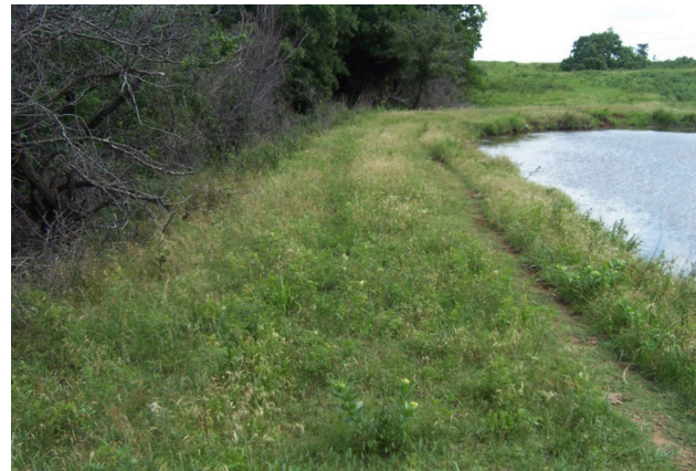
Figure 10. A dam with gently sloped faces and a broad top (top image) and another (bottom) with less favorable slopes and narrow top width, that is experiencing some wave erosion and the beginnings of shoulder damage. Image on left courtesy Alabama Cooperative Extension Service.
