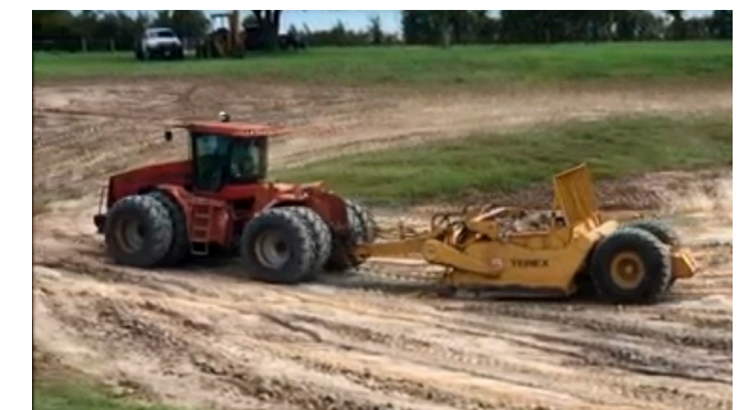
Figure 2. Pond contractors often remove soil from the basin area by scraper, which then is used to lay in 6-inch thick "lifts" to construct the embankment (dam). With proper moisture content and a sheepsfoot roller or dozer tracks, adequate compaction is achieved. An all-wheel drive tractor is an efficient equipment option often used by earthwork contractors doing pond work.
